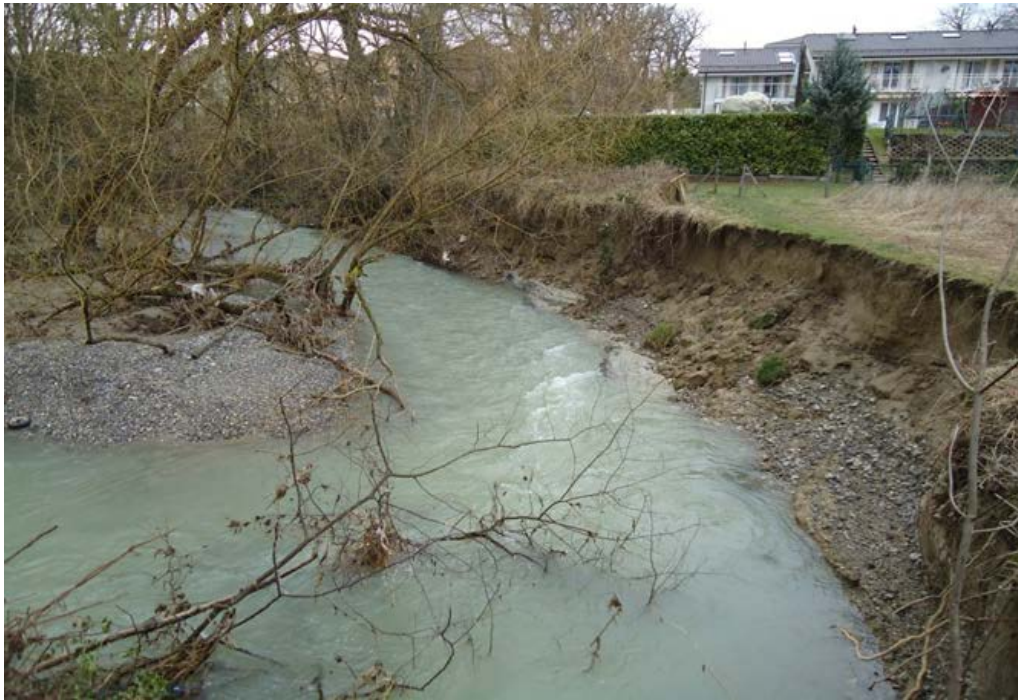
Figure 6 Unstable bank at around 4km of the D/S end (Photo taken on 4.03.2014).
